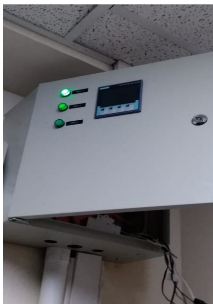
Figure 15 – Slave node (PAC 3100) in electrical cabinet
